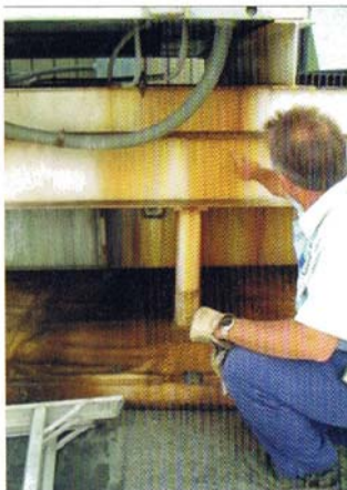
Refrigerant leaks are common maintenance problems.
